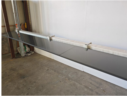
Window Eave Sun Shading
